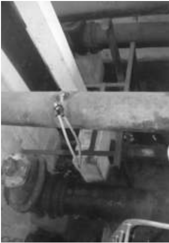
Figure 4 East reservoir Inlet and Outlet
